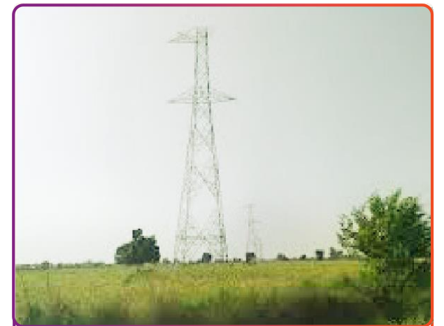
765kV Ghatampur TPS-Agra SC line
