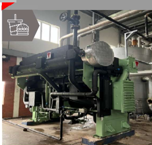
Recently commissioned a 220 TR steam fired vapour absorption chiller for a leading palm oil producer in Malaysia
