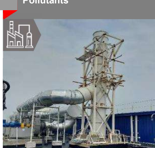
Commissioned a process exhaust system for 2 GW solar cell and module manufacturing
