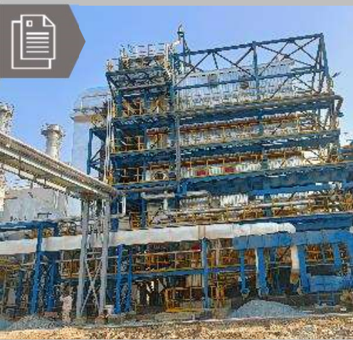
Commissioned a 35 TPH solid fuel-fired boiler for a paper mill in Dubai
