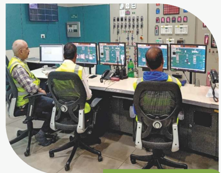
WHR Control Room
