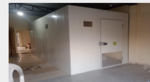
Cold Storage Unit (sangola)
