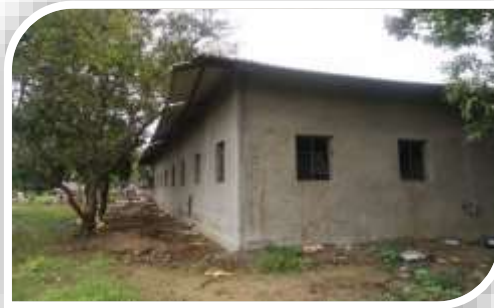
Reconstruction of hostel facility and school for tribal students with Manav Kalyan Trust
