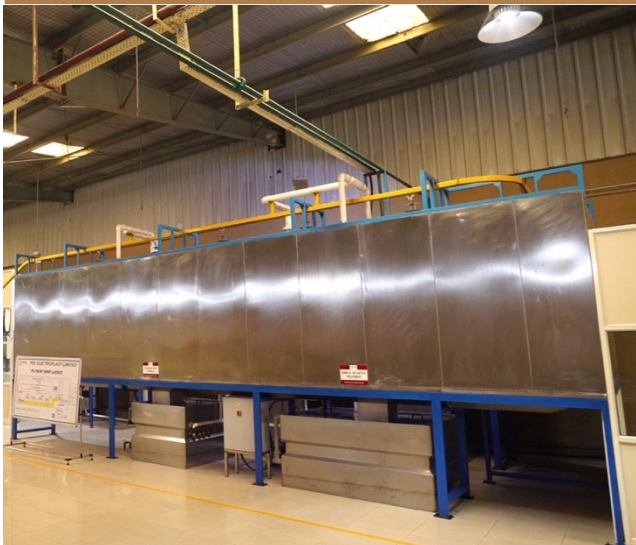
Gas Fired Baking Oven
