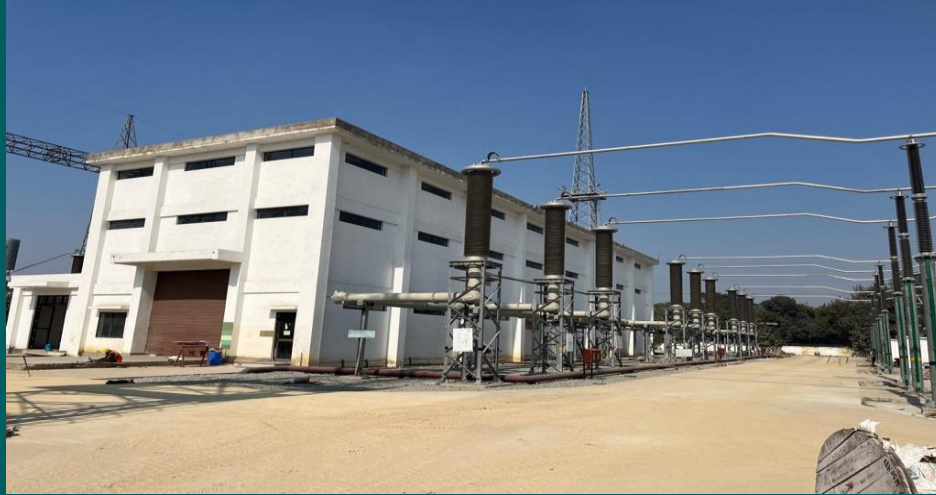
220 kV GIS Substation at UPPTCL Sahupuri
