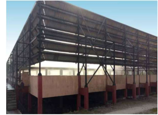
Mist Cooling System
