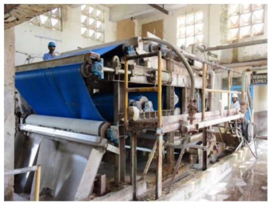
Sludge Handling - Paper
