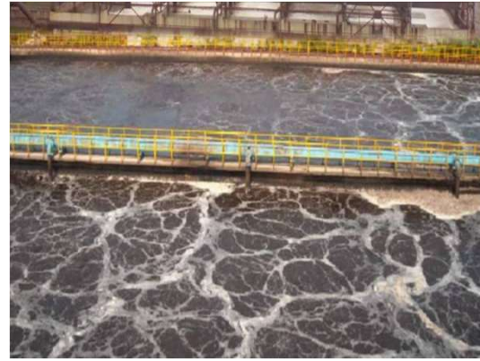
Diffused Aeration System
