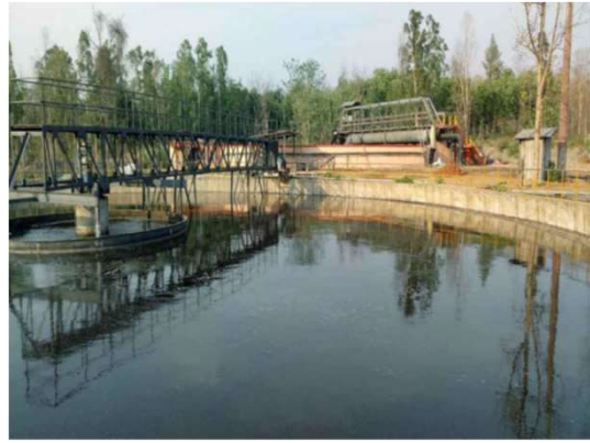
Secondary Clarifier - Pulp
