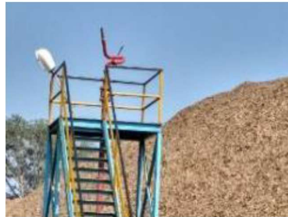
Fire Hydrant Point near chipper
