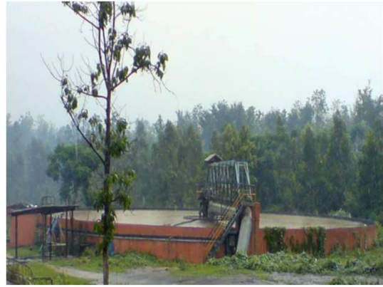
Primary Clarifier - Pulp
