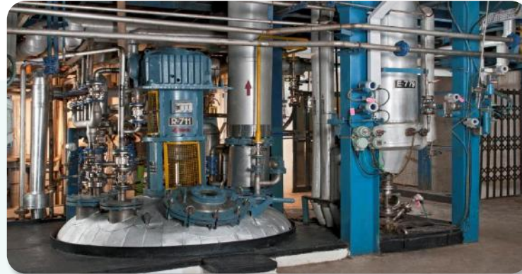
Agro Chemical Plant - Panoli
