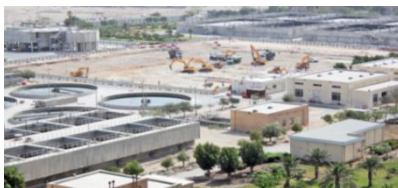
Water Treatment Plant, Doha
