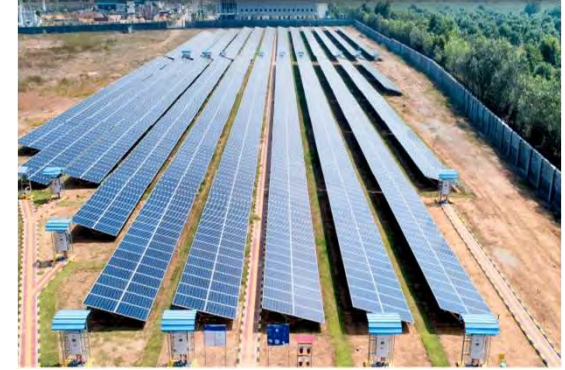
1.3 MW Solar Plant at Sricity
