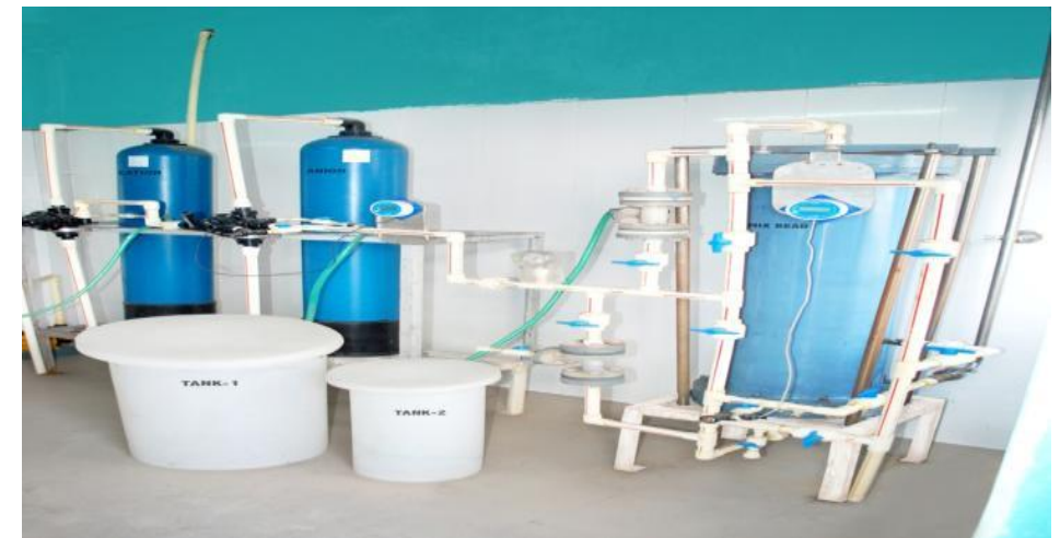
(De-mineralised Water Plant)
