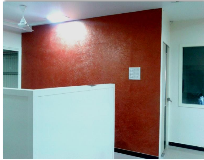
Wall Paneling - (V-Board)
