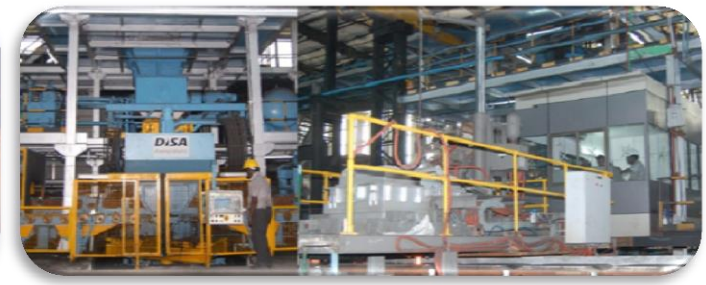
DISA Flex 70HS & DISA Flex 90 High Pressure Moulding Lines & Inductotherm Visipour Tundish, Gudur Plant
