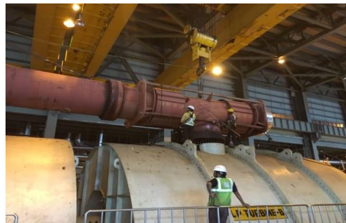
Turbine AOH, 600 MW, Udipi
