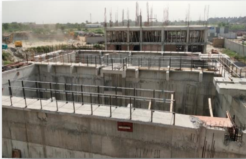
27.5 MLD STP, Networking at Palwal, MCPALWAL
