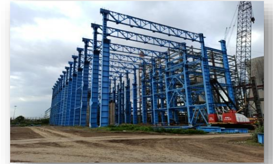
1X660 MW Bhusawal TPS at Maharastra-MAHAGENCO
