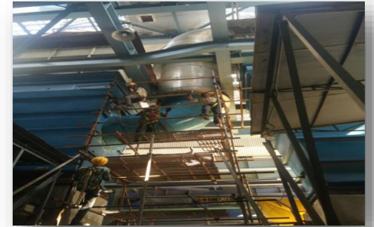
MSH Line Modification, 600 MW Singareni
