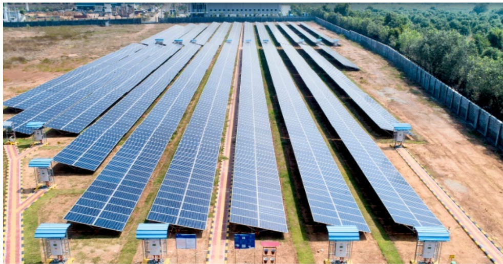
Solar & Wind Installations across plants
