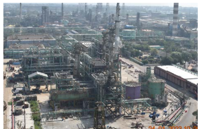
BS-VI SRU Overview
