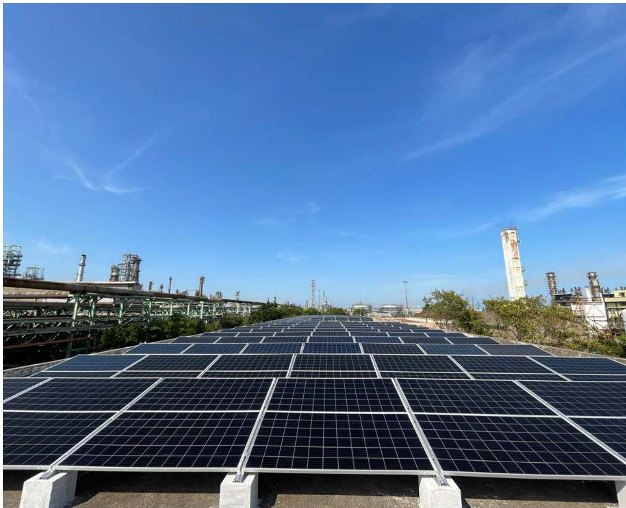
Solar Roof Panels in SS-2
