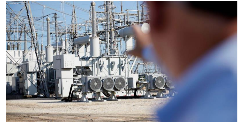
Seven substation projects commissioned, including a remote commissioning
