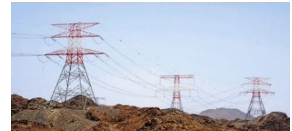
Transmission Lines, Fujirah, Dhaid
