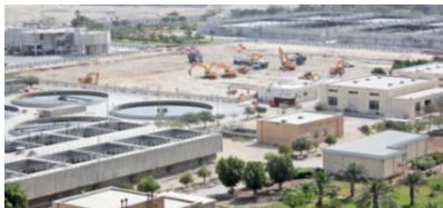
Water Treatment Plant, Doha
