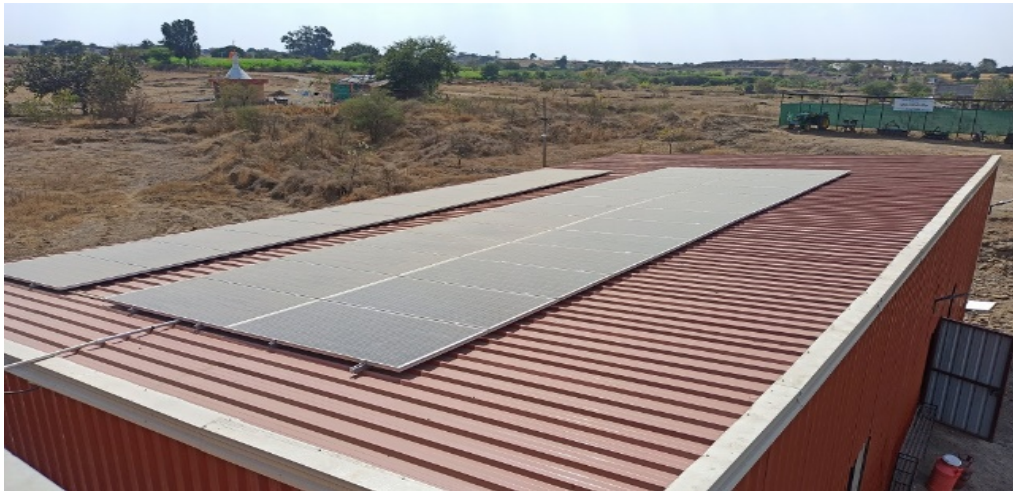
Solar Power Generation at Snehalaya NGO
