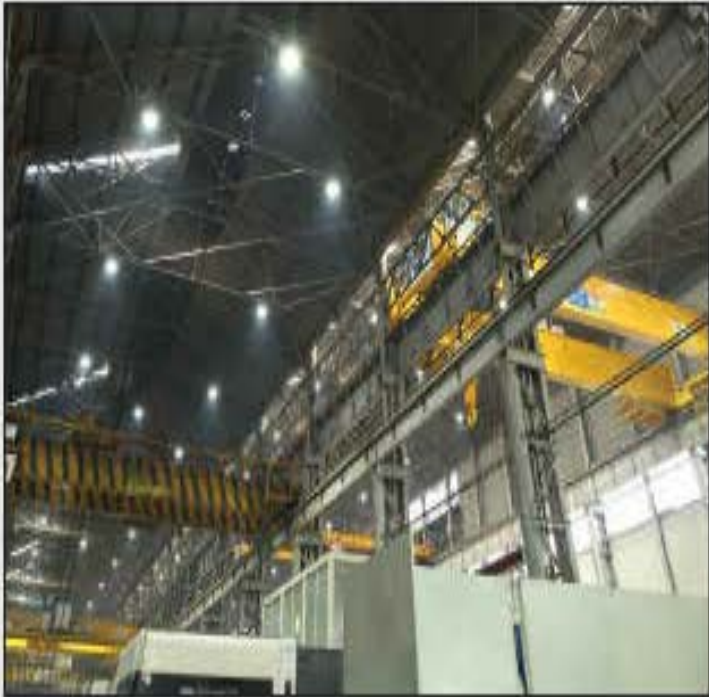
LED bulbs in Offices & Shop floor
