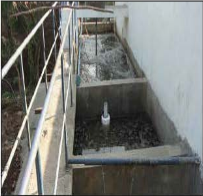
STP Plant for Reuse of treated water
