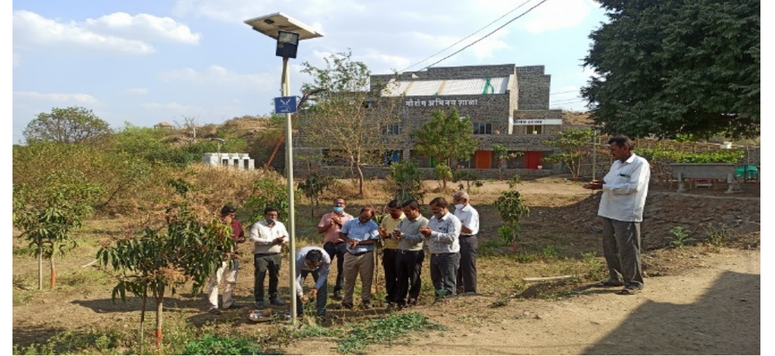
Solar Street Light at Anamprem NGO, Ahmednagar
