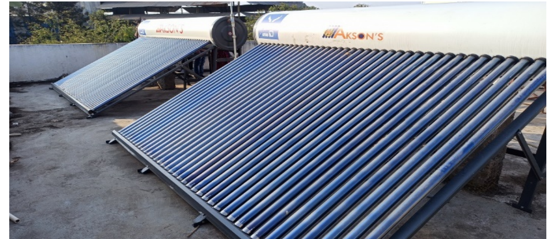
Solar Water Heater units at Snehalaya NGO
