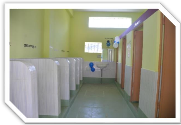
Toilets Constructed in Schools- West Bengal & Haryana
