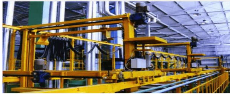
Power handling system for paint shopfloor
