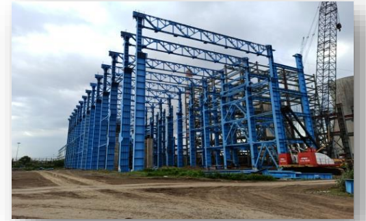
1X660 MW Bhusawal TPS at Maharastra-MAHAGENCO
