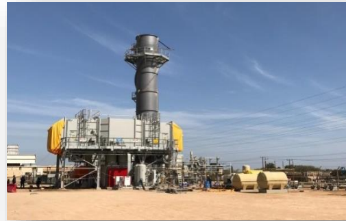
25 MW, Ray Project-RAY International LLC, Oman
