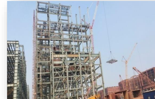
5x800 MW Yadadri TPP, TSGENCO
