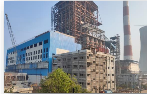
1x800 Mw TPSS, North Chennai, TNGEDCO
