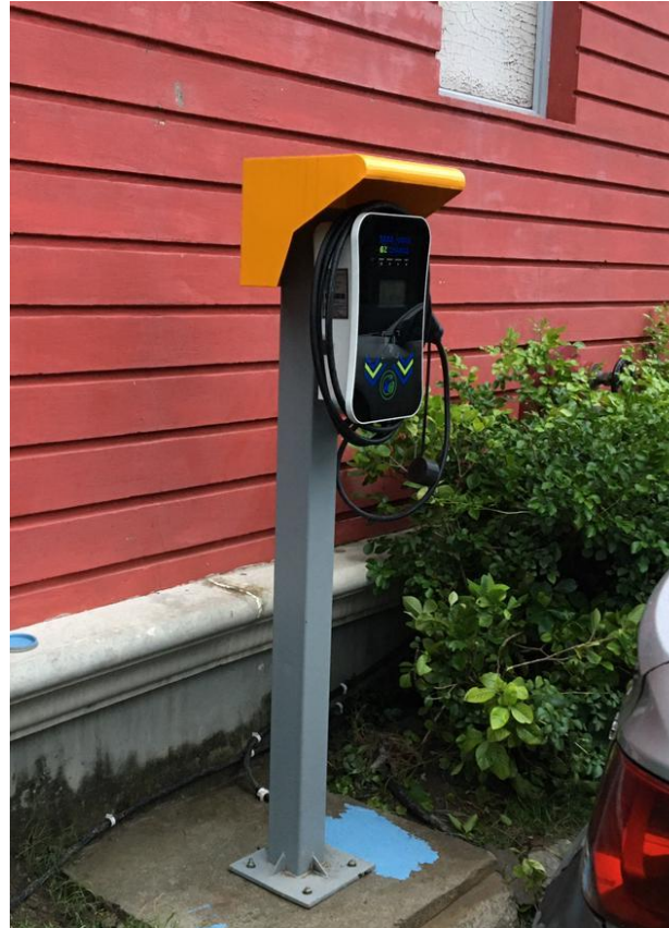
225+ EV charging points installed across ~100 hotels
