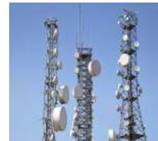
5G Telecom Towers
