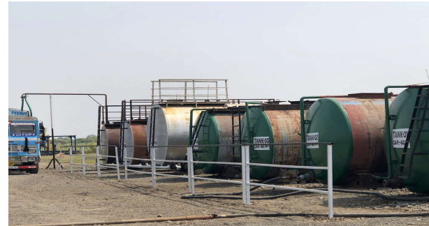
Jyoti I – Oil Storage
