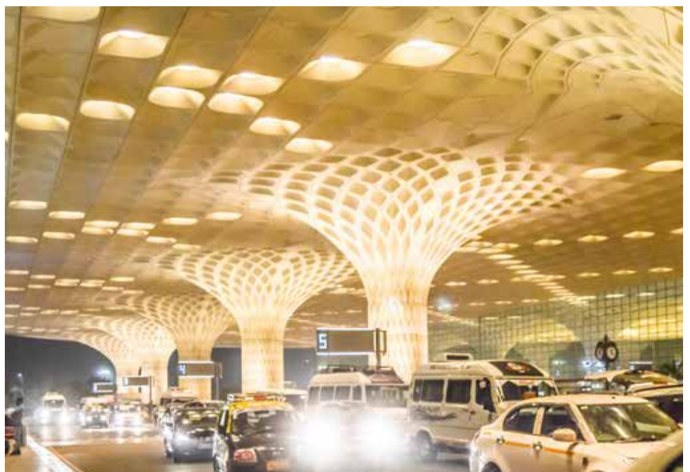
Low and medium voltage solutions for large international airports in North and West India
