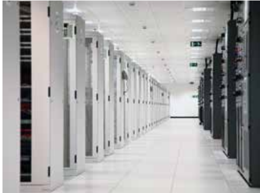
Power distribution and management solutions for the biggest data center majors in the country
