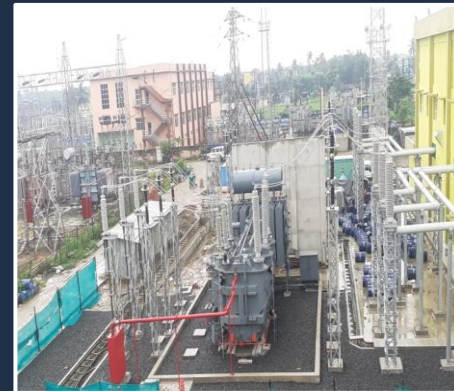
7x220 kV GIS bays, 1x160 MVA ATR, 1 X132 kV AIS Bay charged for DVC at Burdwan
