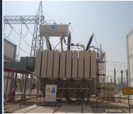
5x220kV AIS Bays, 3x33kV Switchboards with 3x125 MVA Transformers for 300MW Solar Plant evacuation commissioned for Surya Urja at Bikaner
