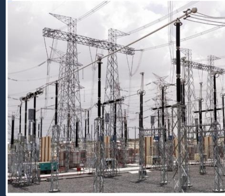
2x765kV AIS Extension Bays with 7x 80MVAR Line Reactors charged successfully for Adani BKTL at Bikaner
