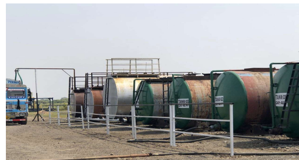
Jyoti I – Oil Storage
