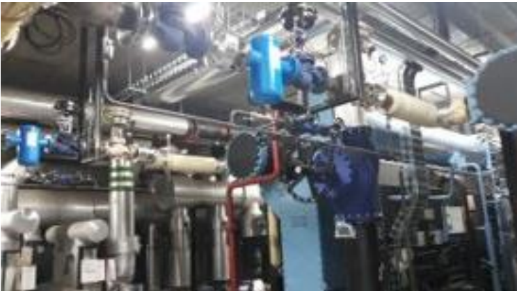
2*813 TR chillers commissioned remotely for a Spanish customer for process and comfort cooling
