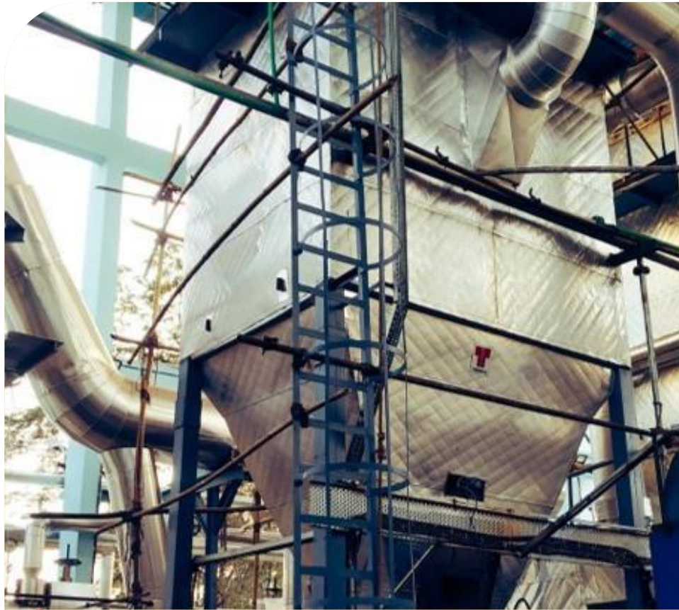
Pulse Jet Bag Filter (PJBF) for a customer in the pharmaceutical industry, installed on a biomass fired boiler
