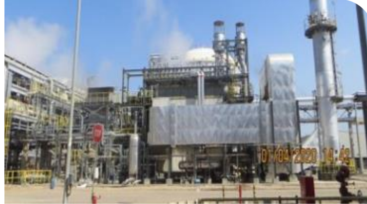
Remotely commissioned large capacity FM boiler in Egypt
