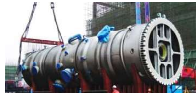
Coal Gasifier for China
