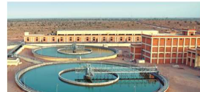
Water Treatment Plant, Barmer
