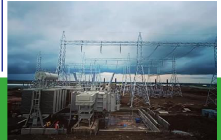
220 kV Switchyard, Khandwa
