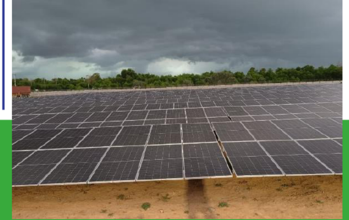
Daiki 2MW solar plant, Sricity, Andhra Pradesh
