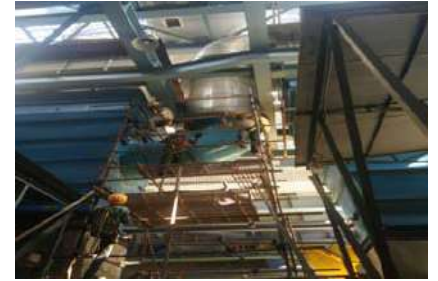
MSH Line Modification, 600 MW Singareni
