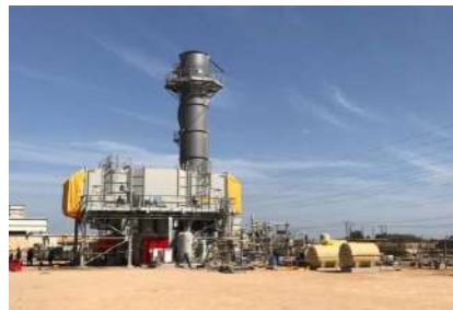
25 MW, Ray Project-RAY International LLC, Oman
