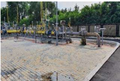
Station Piping at Ennore, IOCL
