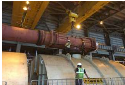
Turbine AOH, 600 MW, Udipi
