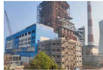
1x800 Mw TPSS, North Chennai, TNNGEDCO
