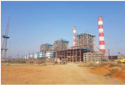
3x660 MW Nabinagar STPP, NPGCL
