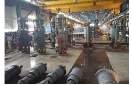
Control & Stop Valves Overhauling Sipat 660 MW
