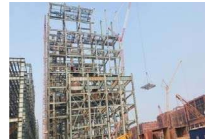
5x800 MW Yadadri TPP, TSGENCO
