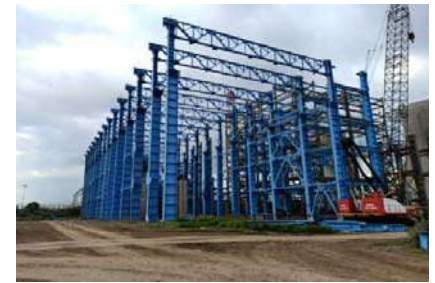
1X660 MW Bhusawal TPS at Maharastra-MAHAGENCO
