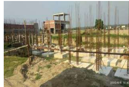
28 MLD STP at Karnal, TPL
