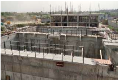
27.5 MLD STP, Networking at Palwal, MCPALWAL
