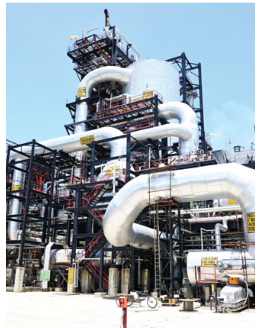
Wet Sulphuric Acid Plant at Haldia Refinery
