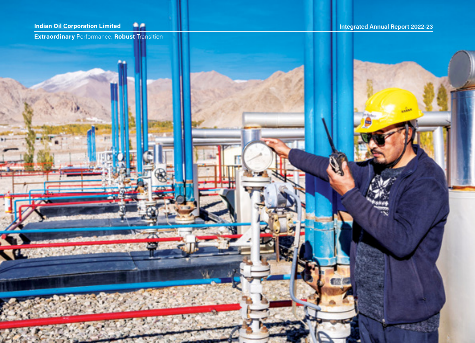
Product pipelines at Leh
