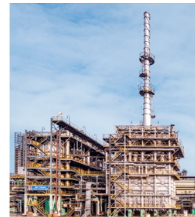
Hydrocracker Unit at IndianOil Panipat Refinery
