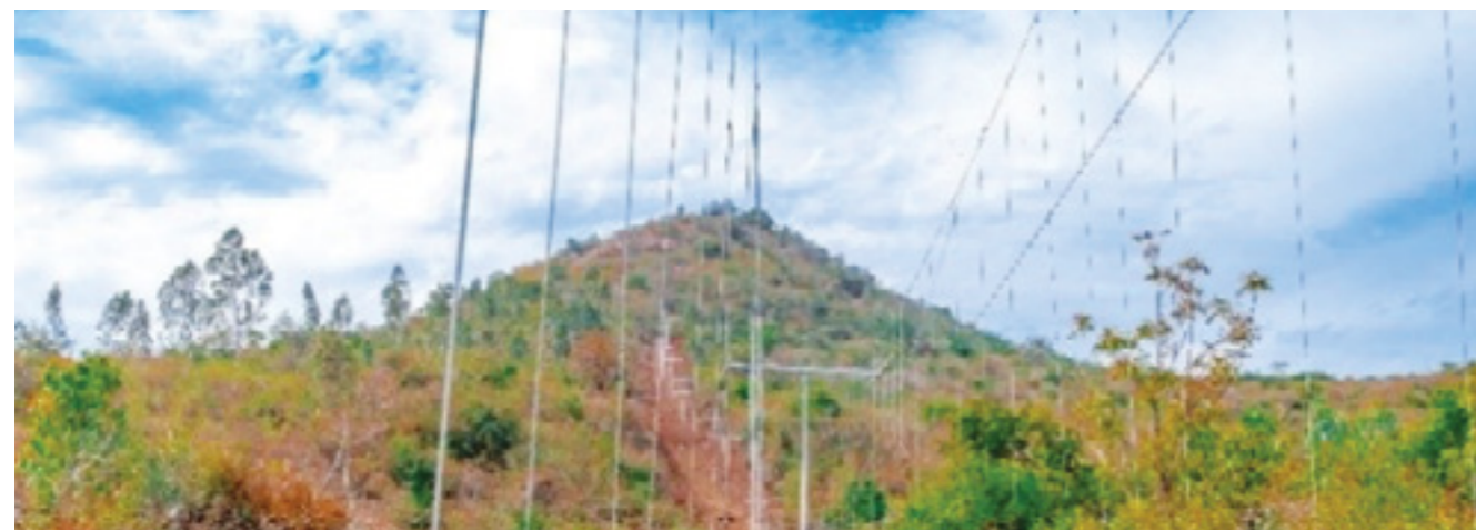
Solar Tentacle Fencing installed at Kaundinya Wildlife Sanctuary, Chittoor, AP
