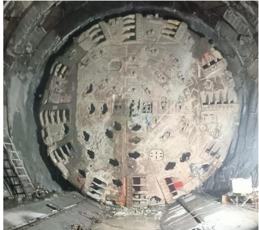
TBM Cutter Head
