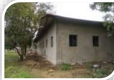
Reconstruction of hostel facility and school for tribal students with Manav Kalyan Trust
