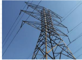
Transmission Line Towers
