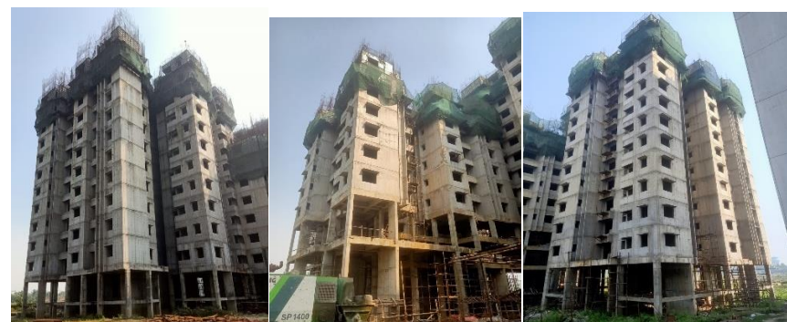
Tower - 22: 12 th Floor in Progress Tower - 23: 8 th Floor in Progress Tower - 24: 12 th Floor in Progress
