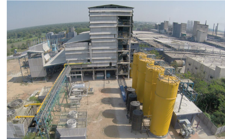
Multiple Effect Evaporator Plant (MEEP)
