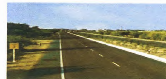
4 laning at Agra- Gwalior section, NH-2, in the State of Madhya Pradesh
