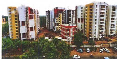
Construction of 222 Flats at Keelandev Tower, Bhopal for MP Housing & Infrastructure Development Board
