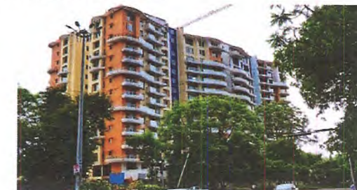
Construction of 96 flats at Tulsi Tower, Bhopal for MP Housing & Infrastructure Development Board
