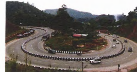
Widening & Strengthening of existing National Highway from 2 lane to 4 lane of Sonapur to Guwahati section of NH-115 (earlier NH 37)
