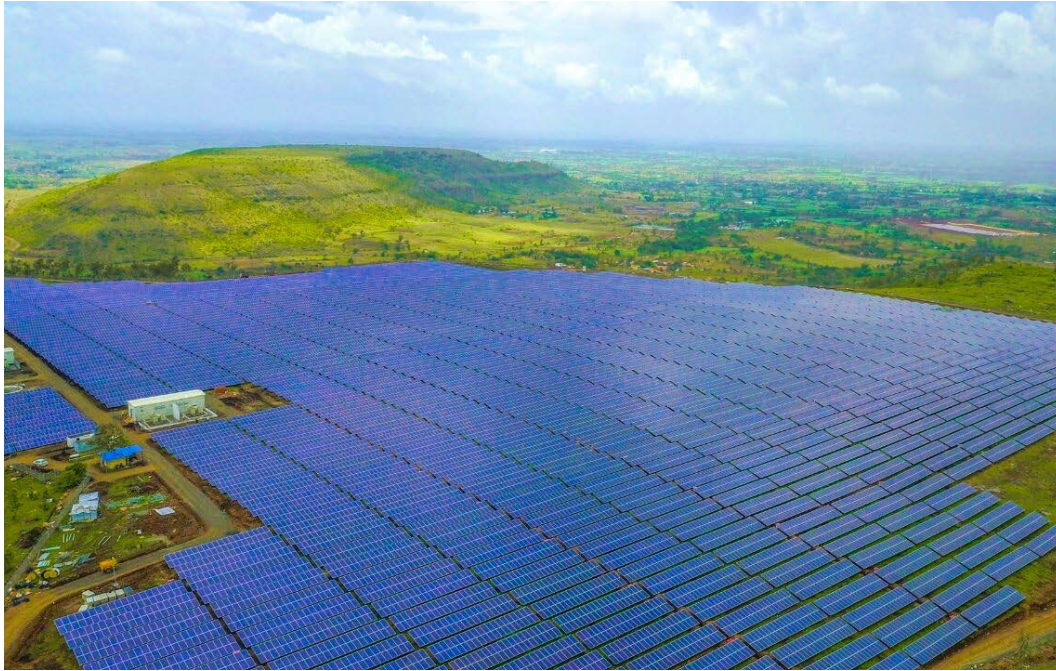
Bagmane Tech Park Belgaum 28 MW ground-based solar project Fastest executed solar project by Bosch
