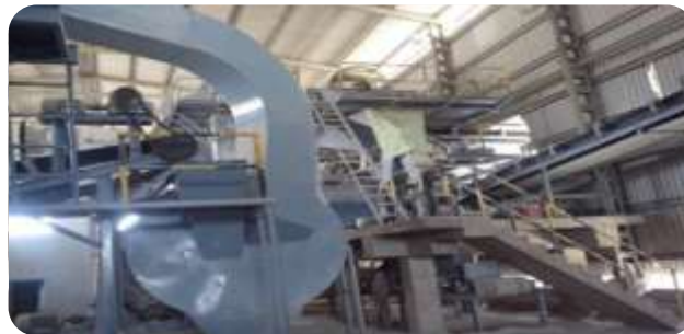
Unit 2– Granulation Plant
