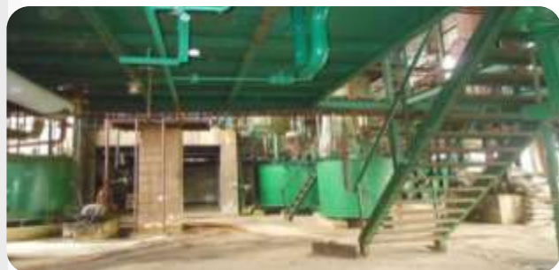
Sulphuric Acid Plant
