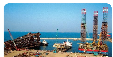
Fabrication Facility, Oman
