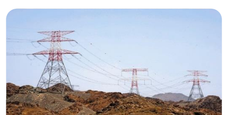
Transmission Lines, Fujirah, Dhaid
