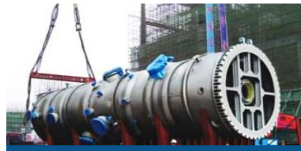
Coal Gasifier for China
