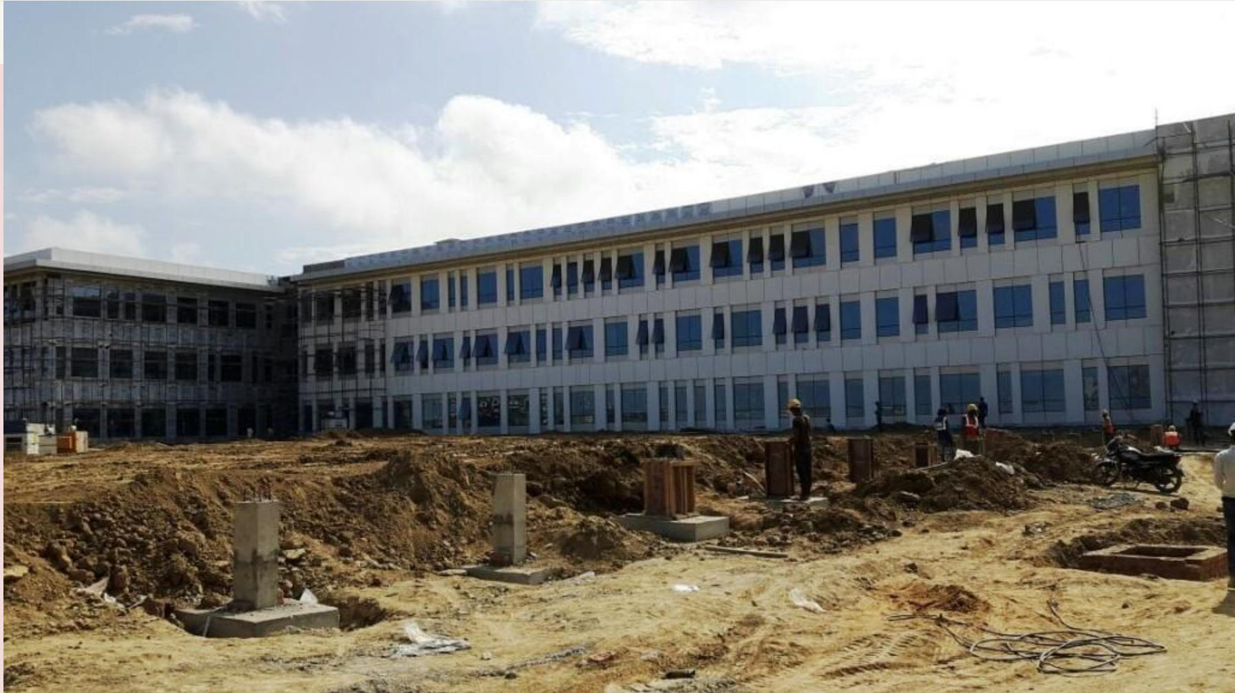
Project of HCL IT City , Chack Gajaria Farms, Lucknow, Uttar Pradesh, Size : 2,00,000 sq feet. Project handed over to customer as per schedule on 6 October 2016.
