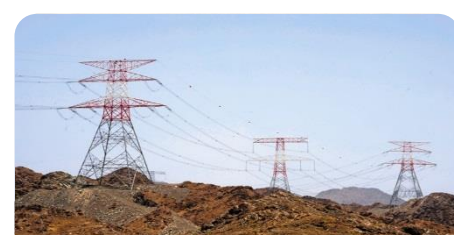
Transmission Lines, Fujirah, Dhaid
