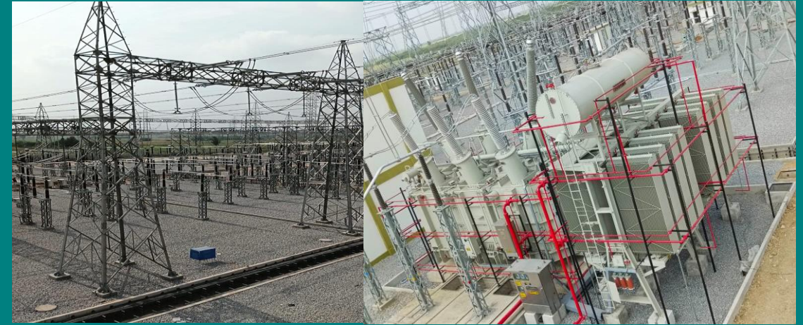
400/220 KV AIS bays at Renew Kopal
