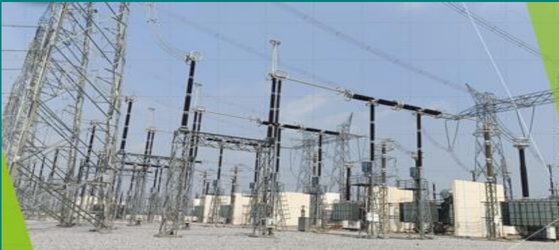
765kV AIS Bays at WKTL Warora
