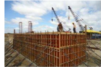
1X110 MW, CIVIL AND STRUCTURAL WORKS ,R&M OF MAIN PLANT, BATHINDA, BHEL (COMPLETED)
