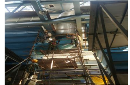
MSH LINE MODIFICATION, 600 MW SINGARENI
