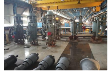
CONTROL & STOP VALVES OVERHAULING SIPAT 660MW
