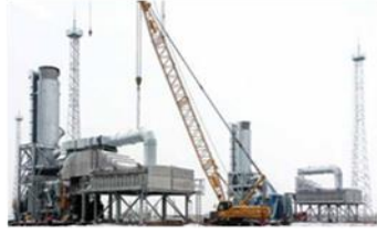
35 MW GT POWER PLANT, KAZAKHSTAN
