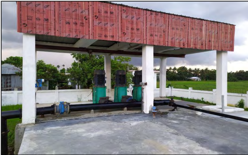
Clear Water Pumps at Rampur, Agartala
