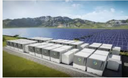
Solar + Energy Storage
